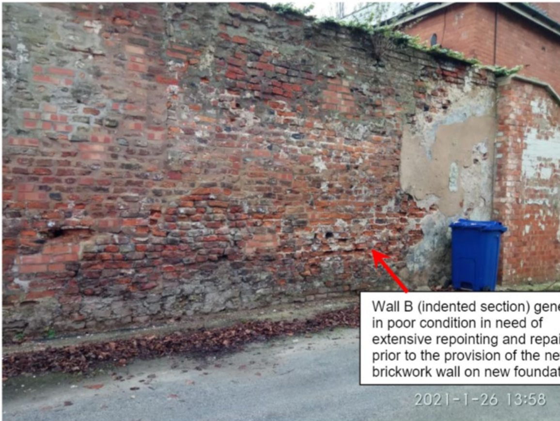
Figure 2: Wall B. Described in the survey as indented with many areas of mismatching brickwork and dilapidated render finishes.
